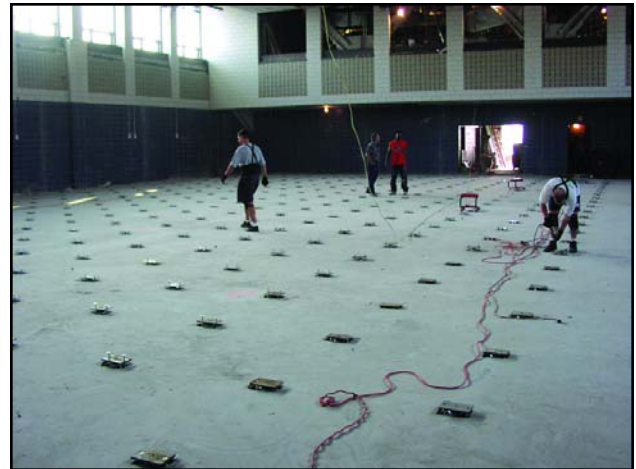
Lifting the slab by screwing down the cover plates and compressing the springs.
