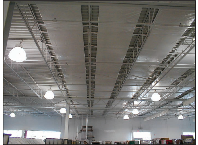
S4 Ceiling Installation in an Industrial Facility
