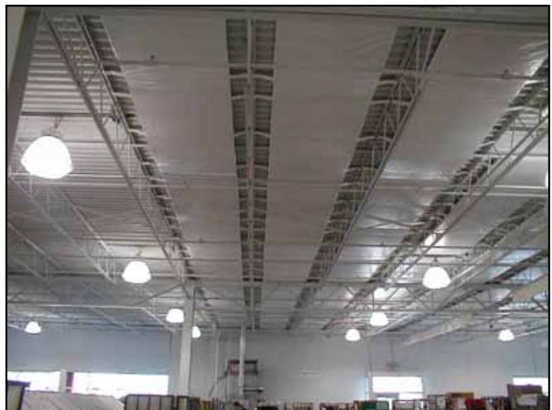
Kinetics model S4 Panel Absorber mounted in the overhead trusses control unwanted reverberant noise to acceptable levels.
