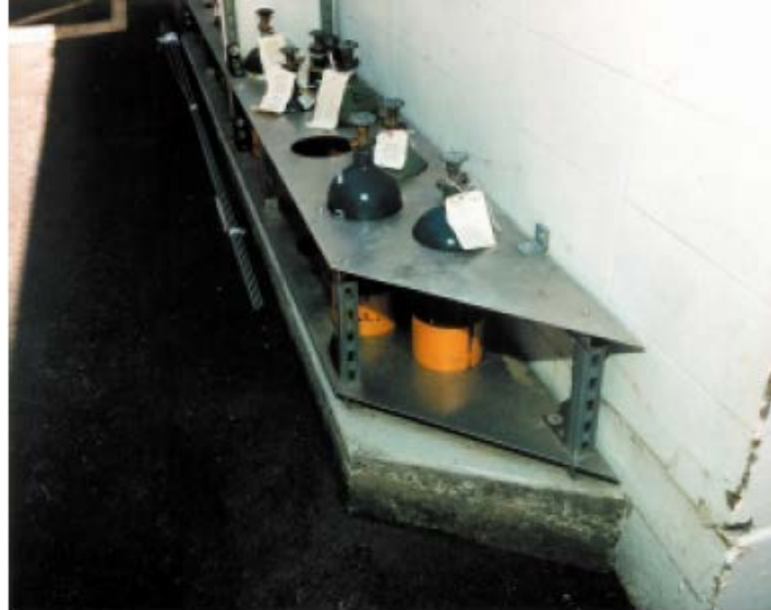
Figure 81: Small gas cylinder storage.
