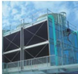
Figure 38: Large cooling tower.
