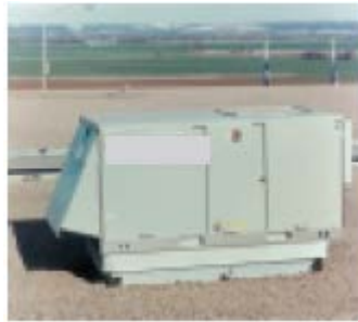
Figure 11: Small rooftop air handling unit.
