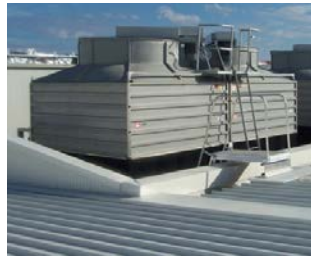
Figure 36: Cooling tower with self-contained sump.
