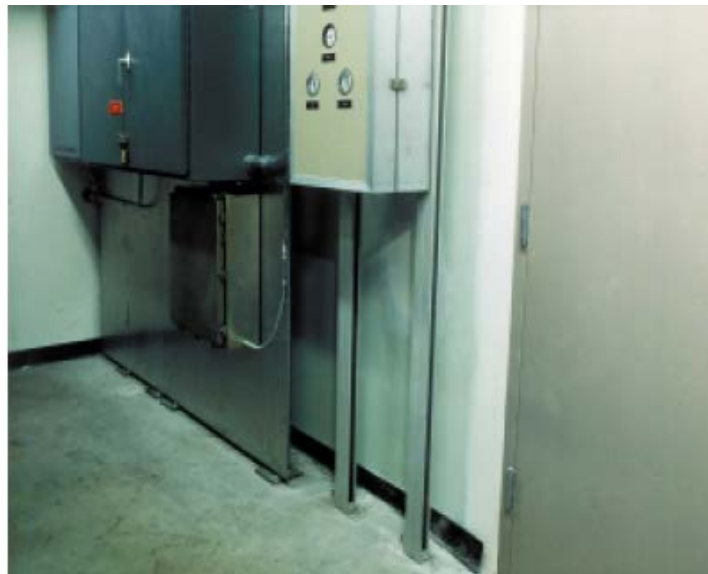
Figure 156: Two different ways to support control panels: using a metal plate attached to floor and ceiling with steel angles (left); using struts extending to floor and ceiling (right).
