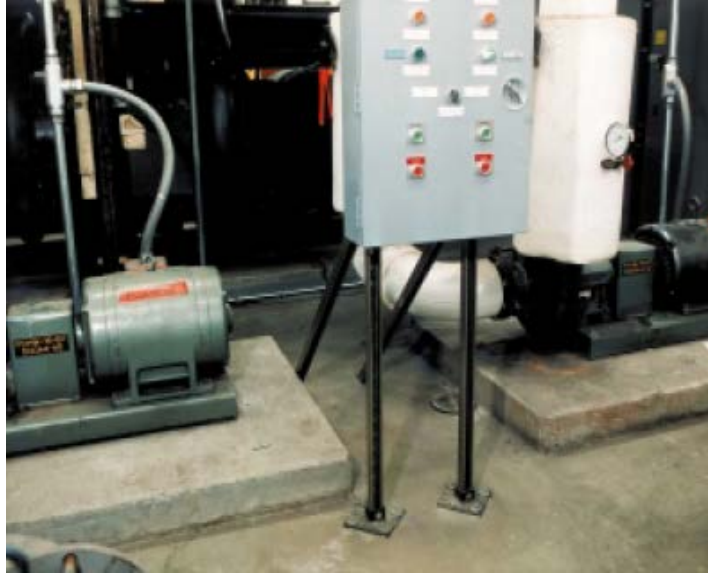
Figure 155: Typical control panel support using angles. Additional angle supports may be required (see below).
