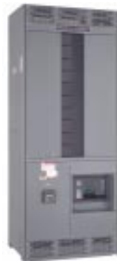
Figure 28: Low voltage switchboard (floor-mounted).
