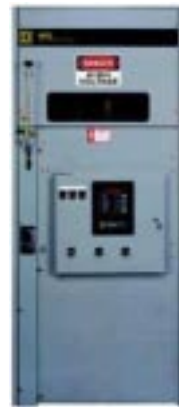
Figure 31: High voltage circuit interrupter (floor-mounted).
