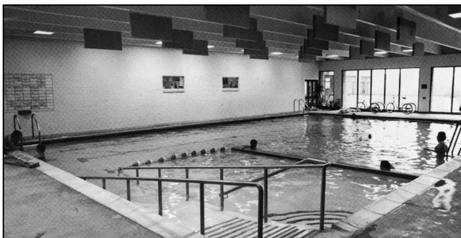
Kinetics decorative acoustical baffles, installed at the therapeutic pool facility at Boulder Memorial Hospital, have helped create a quiet, relaxed atmosphere for physical therapy sessions, fitness classes, and swimming lessons.
