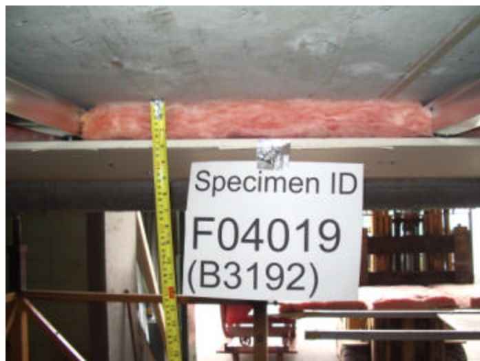
Figure 4: The measured cavity of 76 mm with the insulation and gypsum boards installed on the floor assembly.
