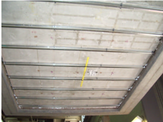
Figure 3: The full view of the IsoMax clips and furring channels installed on the floor assembly.
