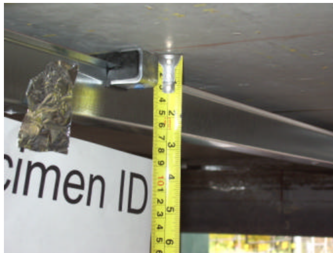
Figure 2: A close view of the IsoMax clip and the furring channel installed on the underside of the NRC reference concrete slab.
